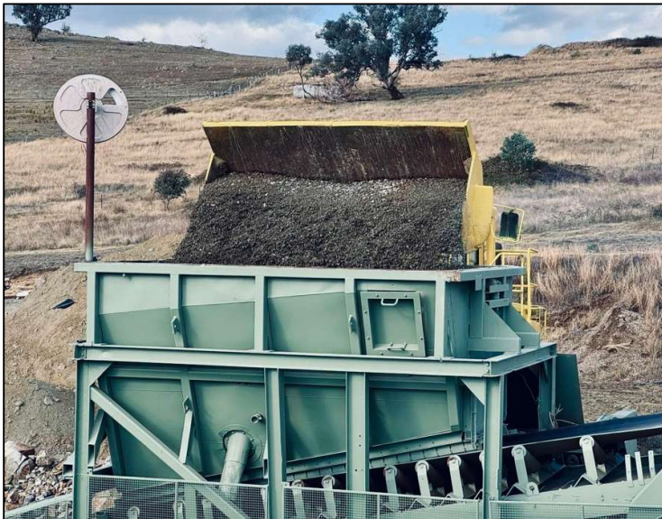
Operating the Challenger Mine processing plant
